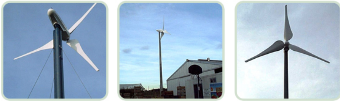
Figures 1,2, & 3 - Images of Grid Link Wind turbines installed across Victoria, Australia
